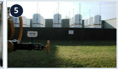
Hydrogen storage area (15 receivers)
