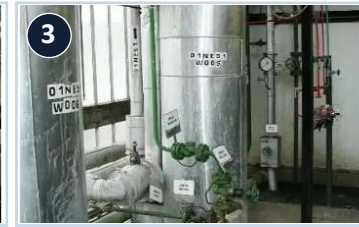
Gas separation & pressure control
