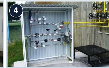
Hydrogen unloading station
