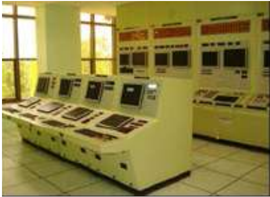
Handling Control Room Panels & Console
