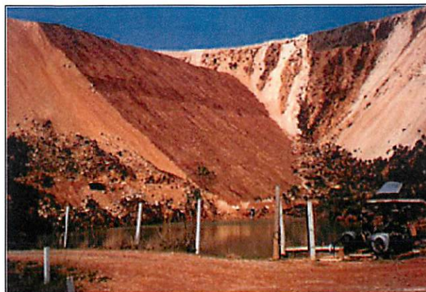
BEFORE: Remediation of an acid-drainage-generating waste-rock dump at the mining site of Pocos de Calcas – Brazil
