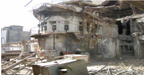
IRT 5000 Research Reactor
