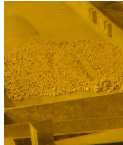
Dried corrosion product
