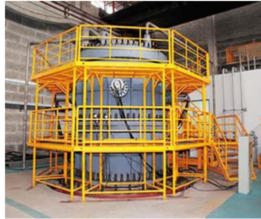
Main Helium Blower
