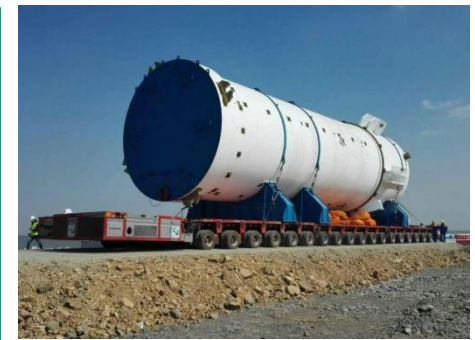
Reactor Vessels Installed
