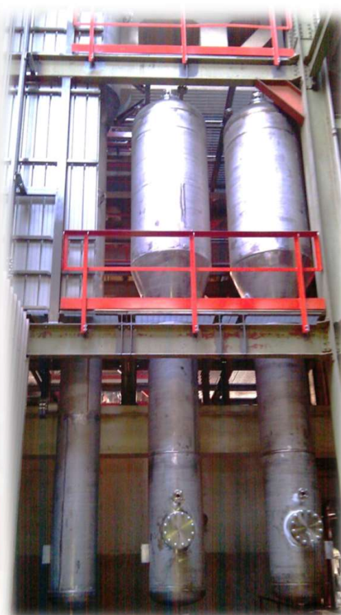
Pressure Suppression pools
