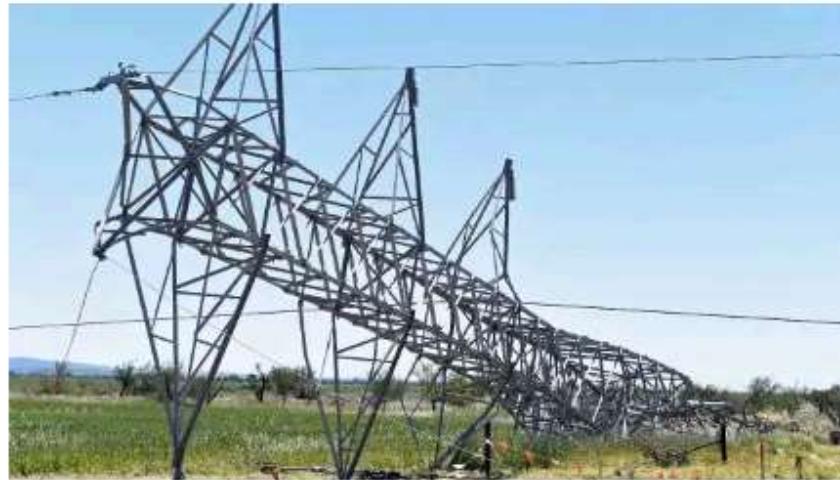
One of the damaged power towers on private property near Melbourne in South Australia. Source: News Corp Australia
