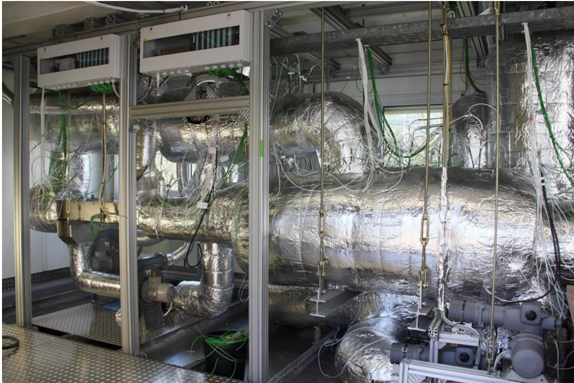
FIG. 2. View of the TELEMAT facility
