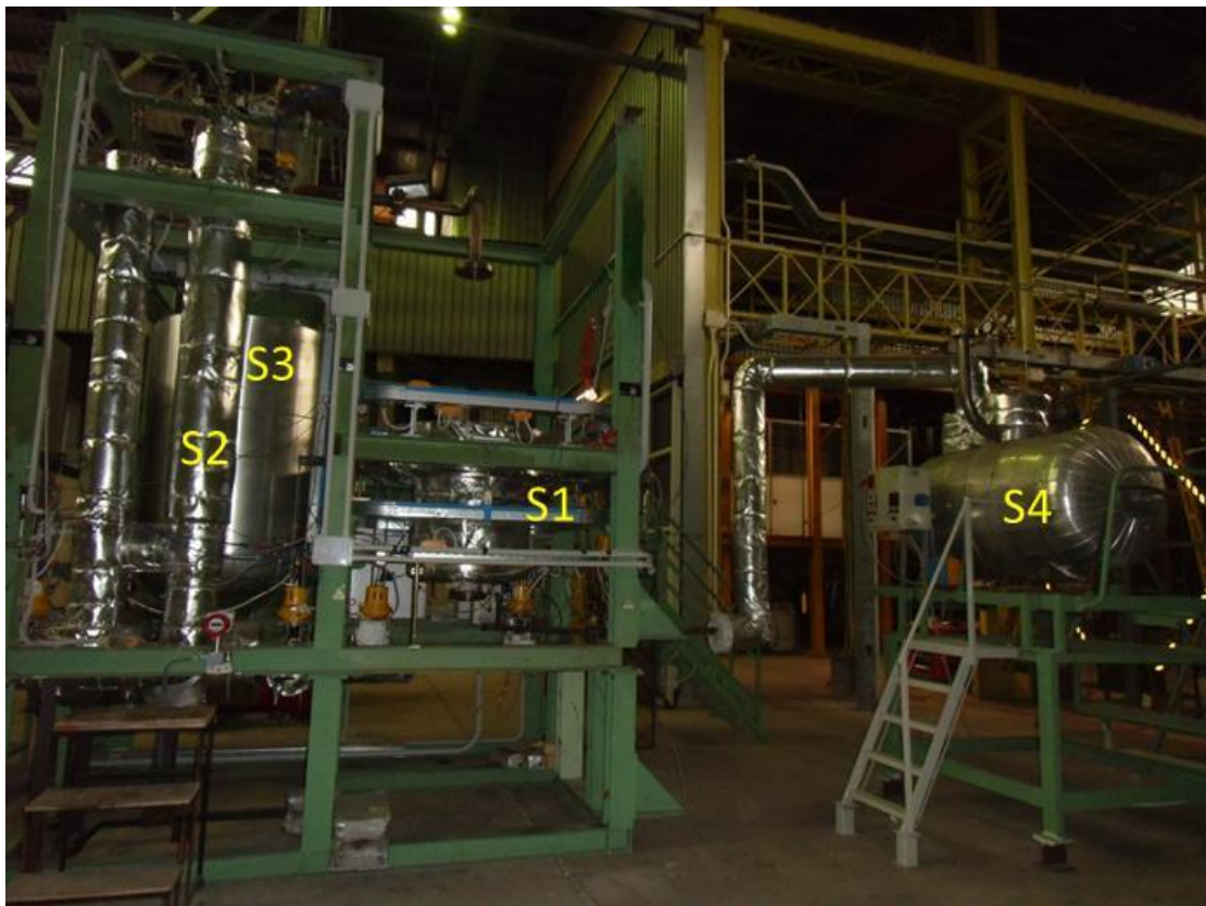
FIG. 3. View of LIFUS5/Mod2 facility.
