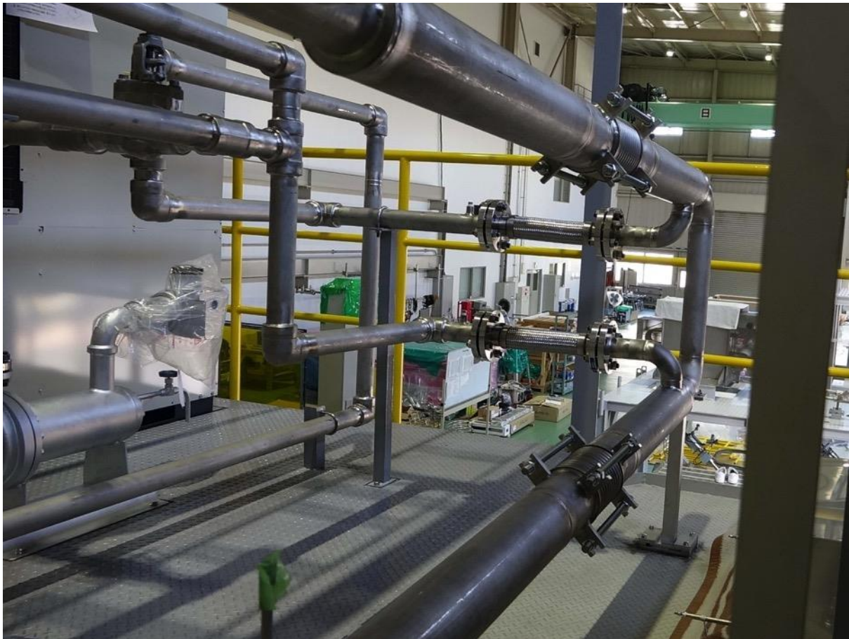
Fig.4 Photo of heat exchanger
