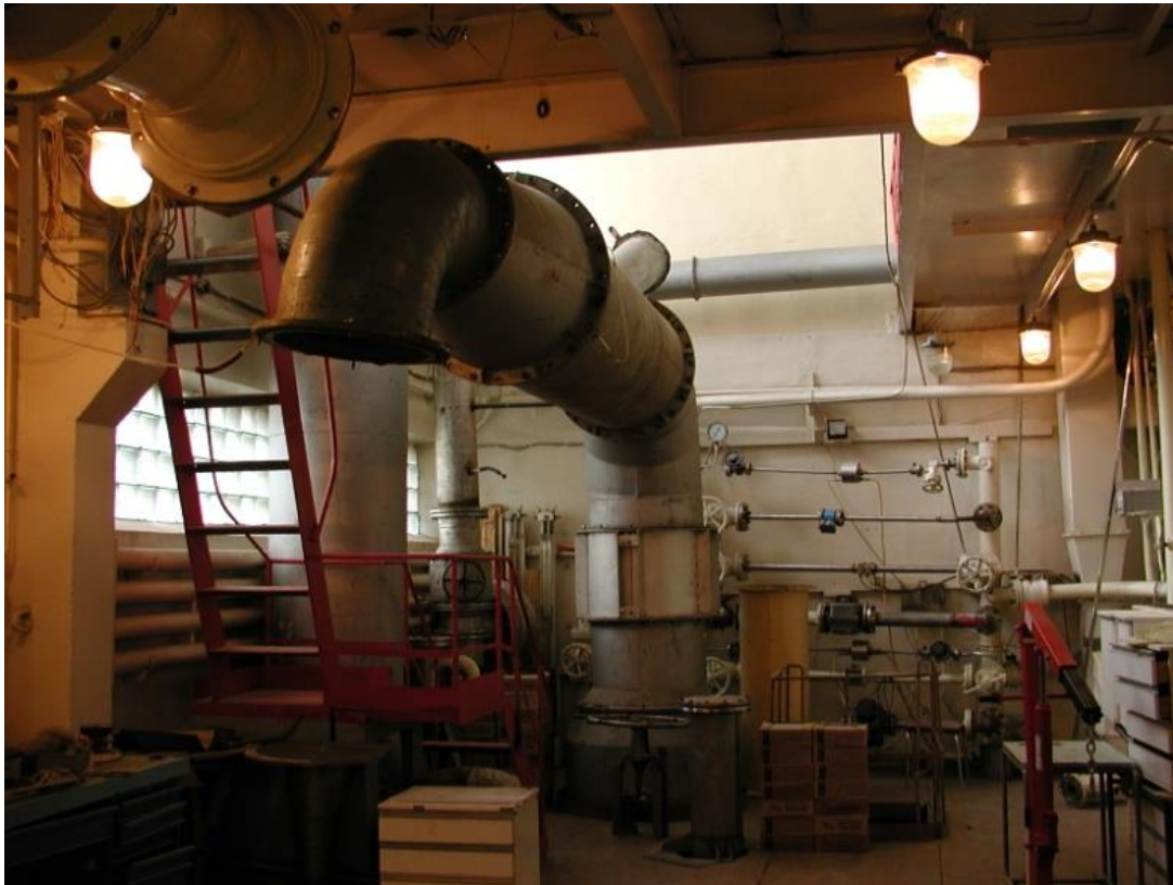
FIG. 2. View of the SGDI facility
