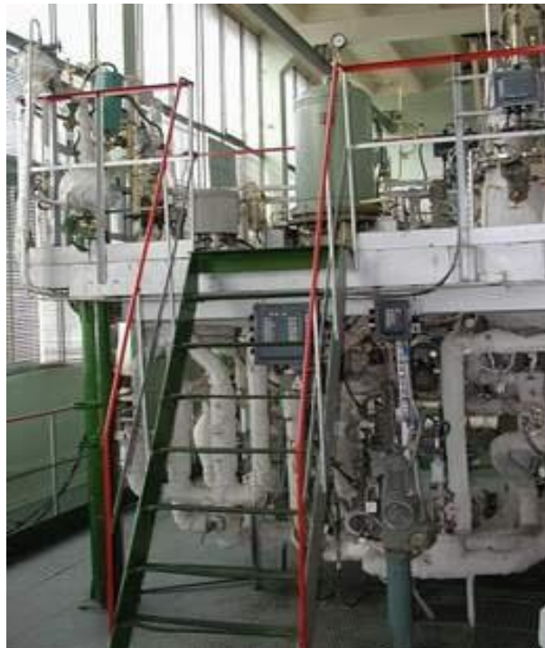
FIG. 2. General View of "TT-2M" Liquid Metal Facility
