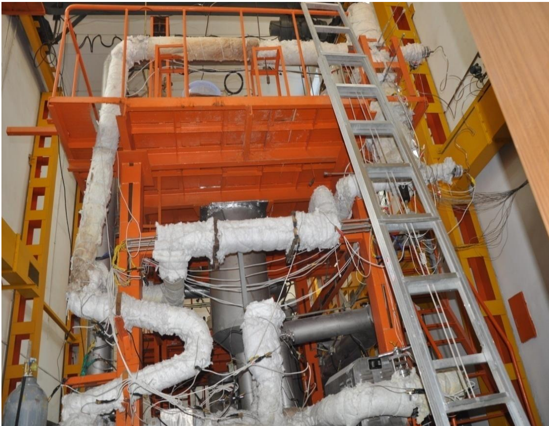
FIG. 4. Photo of the two-phase boiling sodium loop
