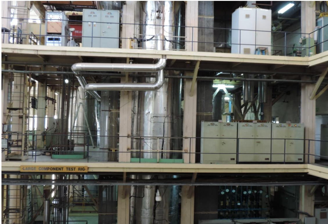
FIG. 2. LCTR Structure with Pipe lines and Test Vessels
