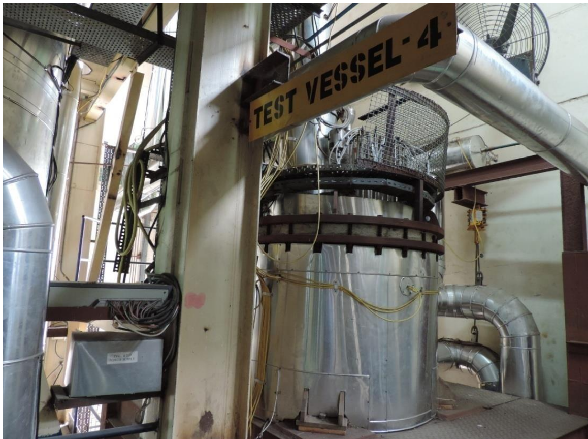
FIG. 3. Test Vessel-4 with Decay Heat Exchanger
