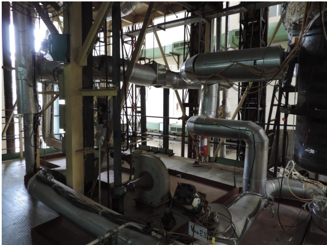
FIG.3. TSTF Loop Pipe lines
