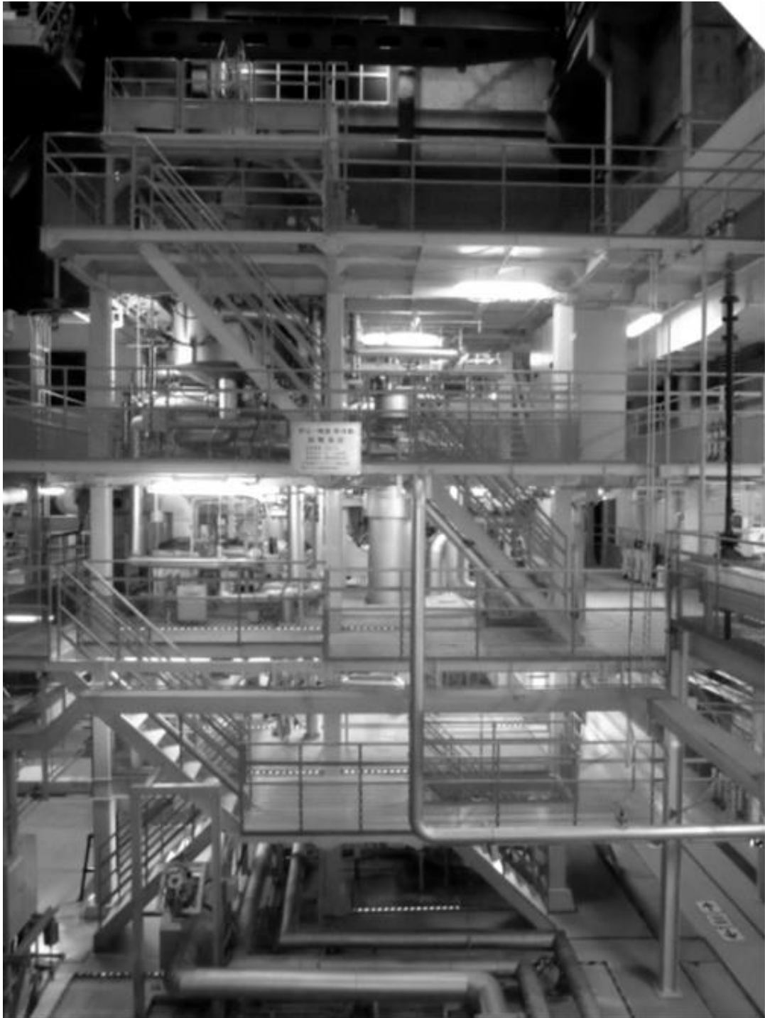
FIG. 3. Panoramic view of CCTL apparatus
