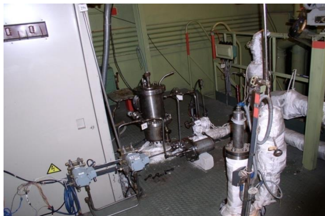
FIG. 2 Overall view of the PLUTON facility (upper platform)
