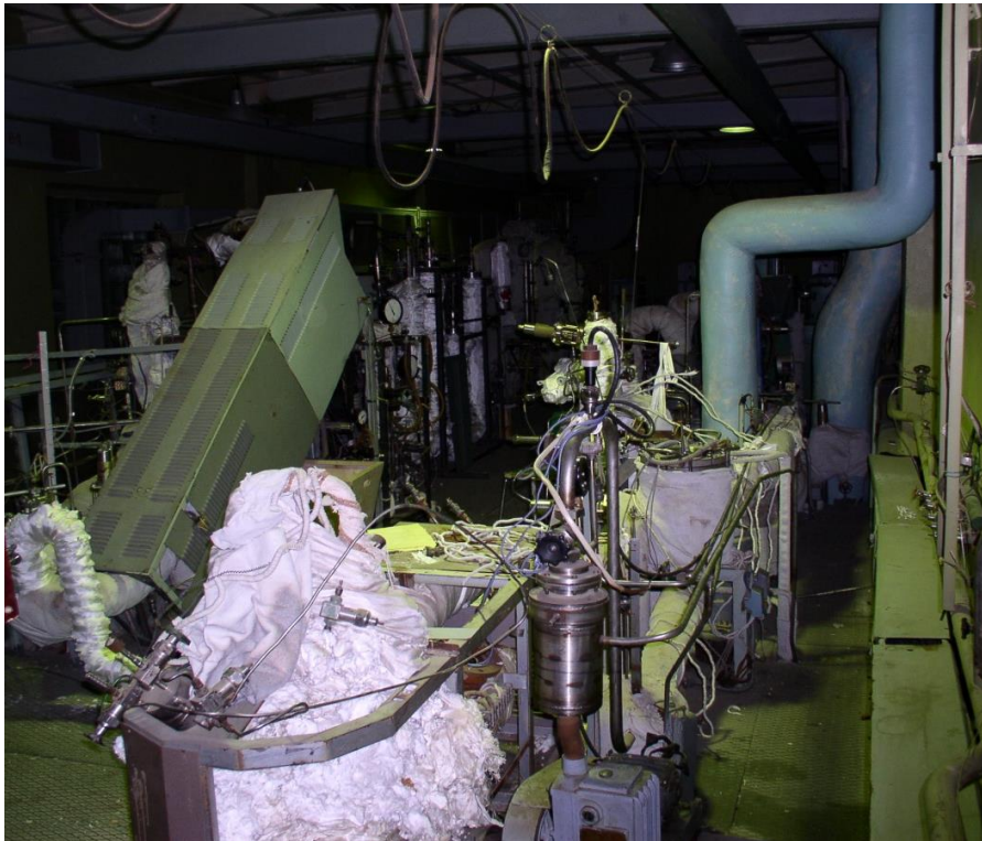
FIG. 2. Protva-1 facility, first level.
