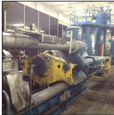
FIG. 1. Views of the Material Processing Facility
