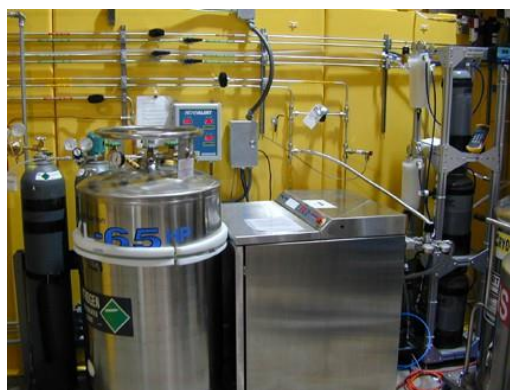
Figure 5. Nitrogen gas, hydrogen generator and deionized water supply.
